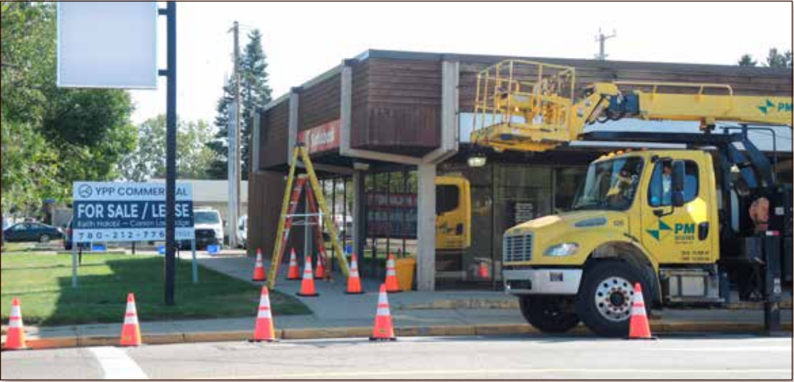
The Bank of Nova Scotia branch in Morinville is now permanently closed. The signs were removed from the building on September 10. - Lucie Roy Photo
