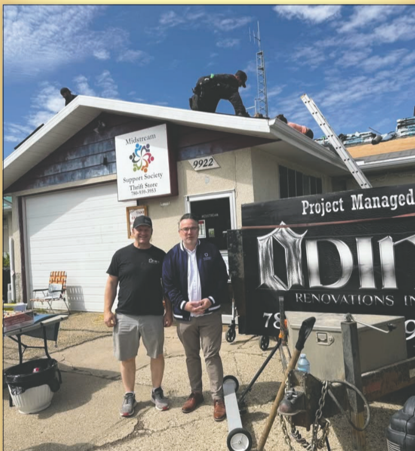
Curtis Farvolden, owner of Odin Renovations Inc. (left), and MLA Dale Nally stand outside the Midstream Support Society building in Morinville as crews work on a new roof donated by the company. The project was completed at no cost to the organization with support from local businesses and volunteers. Odin Renovations Inc. photo
