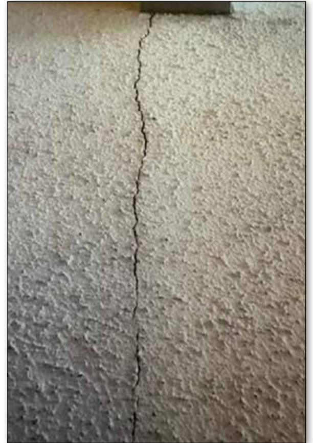
A large crack in the ceiling is one of several areas of damage found throughout the home after the earthquakes.
