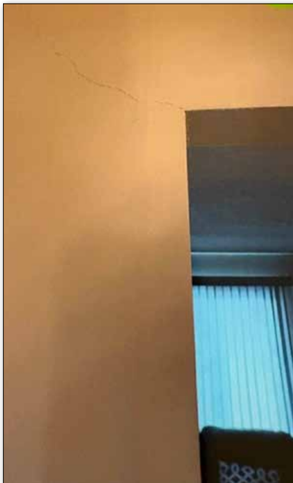
Cracking in the drywall appeared throughout the home following the seismic activity in the area.
