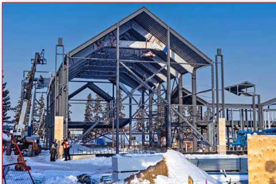
Work was progressing nicely on St. Jean Baptiste Church in Morinville in late December. The church is set to officially open for Christmas Mass in 2025. - Stephen Dafeo Photo
