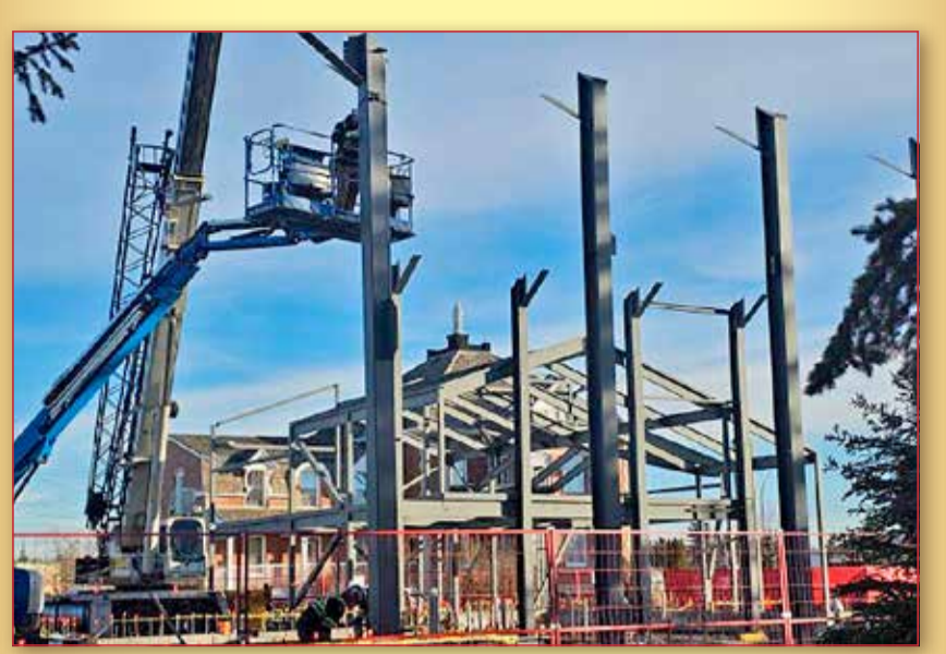
Workers erect the steel frame of St. Jean Baptiste Church on 100 Avenue in Morinville. The church, which was destroyed by fire, is set to reopen for Christmas 2025. - Stephen Dafeo Photo
