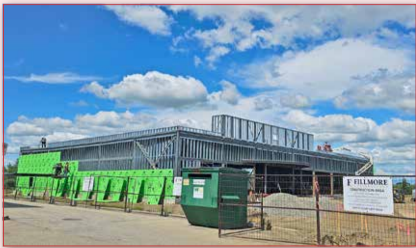
Fillmore Construction is making progress on the new Shoppers Drug Mart location on 100 Street, north of No Frills. - Stephen Dafoe Photo
