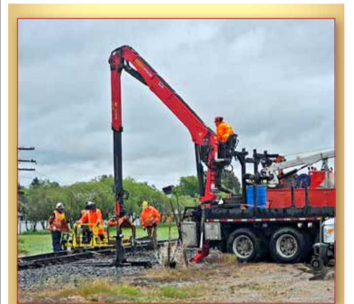
CN workers were out on a rainy day June 12 working on the track at 100 Street. - Stephen Dafoe Photo
