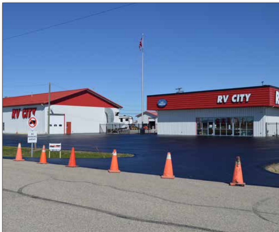
RV City at 8704 100 Street in Morinville is getting a fresh new look! The parking lot was upgraded with new pavement, making it smoother and easier to drive on. This is a great improvement for the business and will make it more enjoyable for customers to shop for their next RV purchase.
