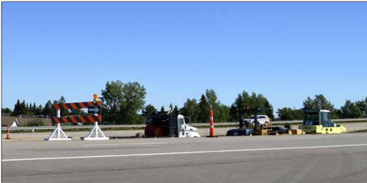
Construction upgrades continued through the week of August 29 on the bridge just outside of Morinville on St. Albert Trail Highway 2. Workers were busy during the hot weather, continuing to get their job done. The upgrades are expected to be completed by the end of September.
