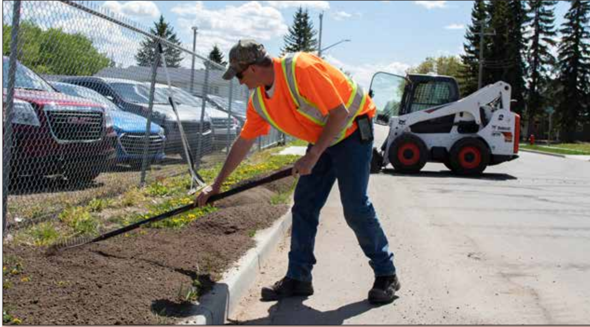
Town of Legal maintenance employee Lorne Witter rakes fresh dirt on the side of 47 Street on June 1. "We're re-landscaping where we had some curb work done," he said. "With the new curbs we're trying to bring it back up so water's not sitting there and perforating it underneath our curbs and cracking them and making more work for us." Photo by Grant Cree.
